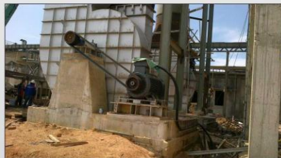
Application - Wet Scrubber ID Fan Customer - Steel Plant, Indonesia FAN - 325HP
