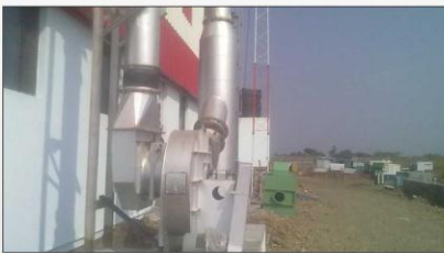
Application - Furnace Exhaust Customer - Mahindra, Chakan FAN - 10HP
