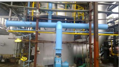
Application - Incinerator Customer - Atul Ltd., Vapi FAN - 15HP
